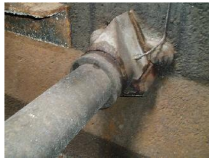
Peak Cap bearing, shaft and grease line
